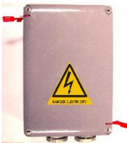
Figure 36: New style service terminal box fitted with tamper proof seals and Danger Electricity sticker.
