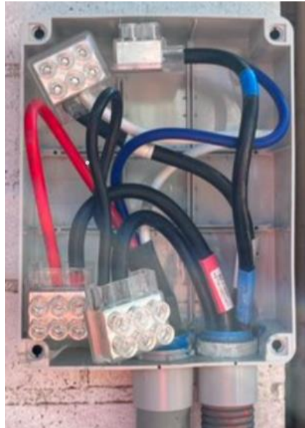
Figure 35: 100 or 200 Amp service termination with terminal blocks
