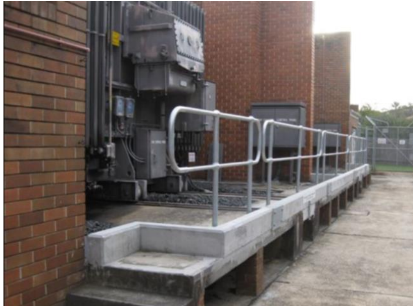
Figure 2: Oil Containment Bund with Gravel
