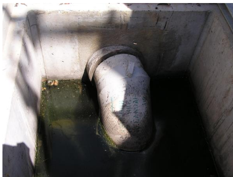
Figure 5: Typical Flame Trap (grate removed for photo)
