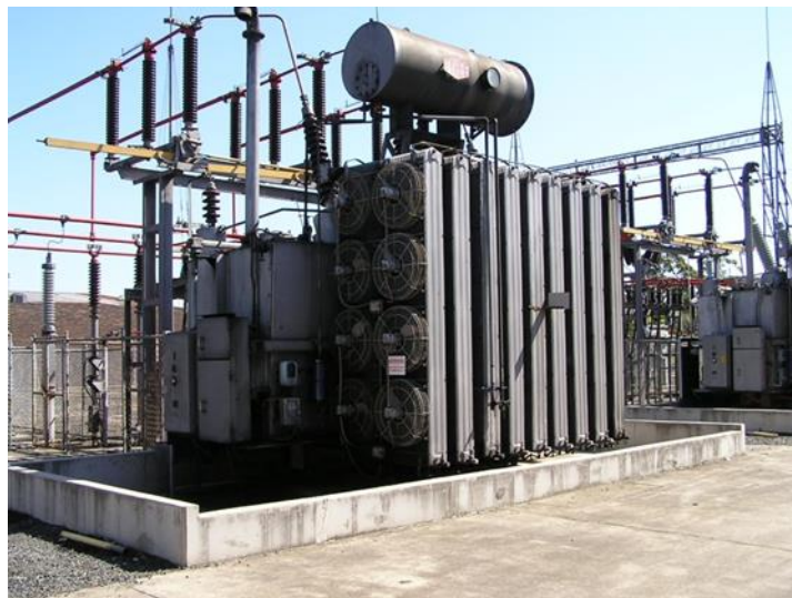
Figure 1: Typical Oil Containment Bund
