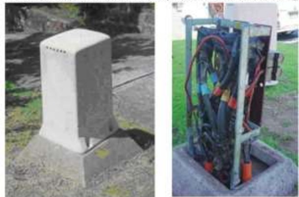
NS199 – Clause 9.3.7 – Steel framed pillars in the lower hunter region
