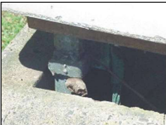
Figure 1 – Typical steel framed pillar (lower Hunter region) (including 50mm opening, for steel frame detection)
