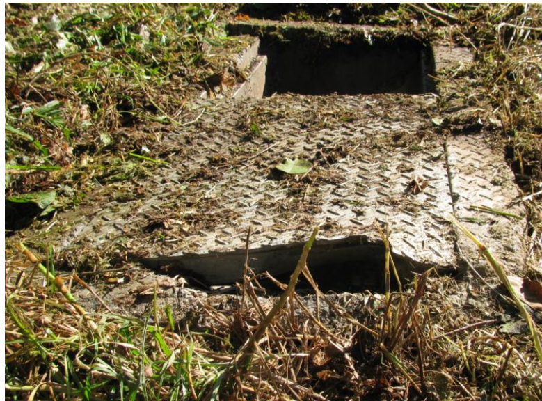
Figure 4 Pit damage – concrete shell broken and lid deformed
