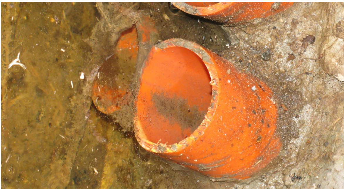
Figure 5 Incorrect conduit entries to a pit
