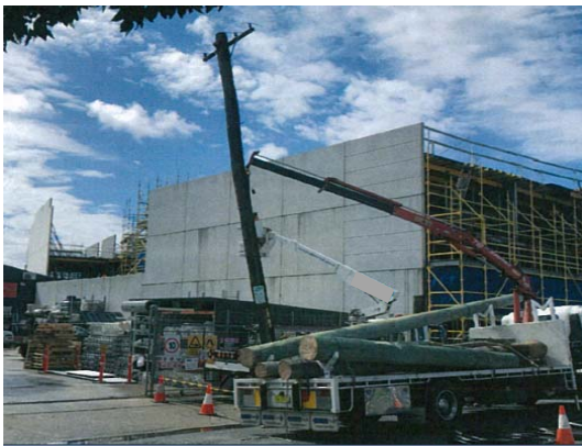
Picture 1 showing pole had failed and was held
