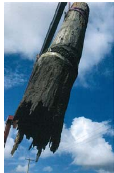
Picture 2 showing pole deteriorated condition
