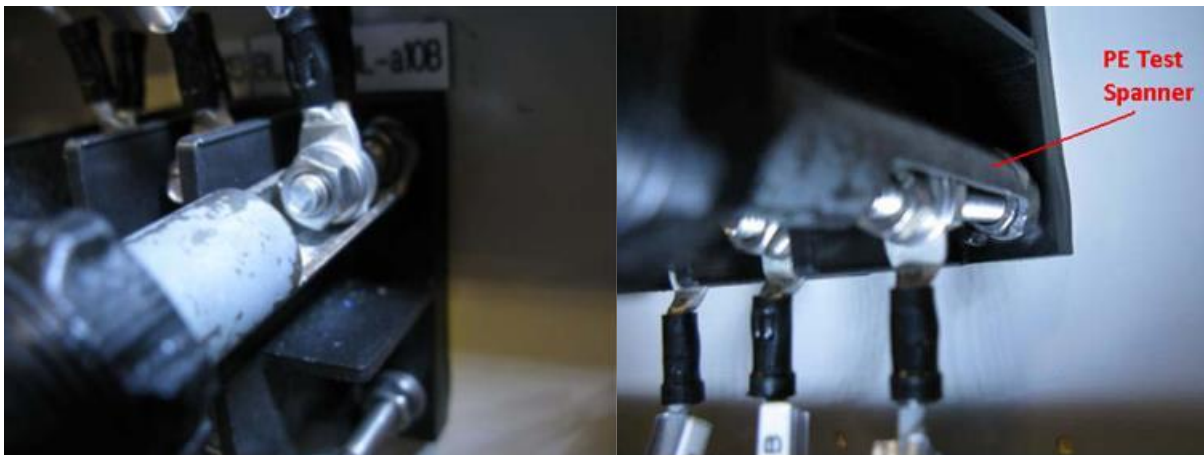
Figure 7: PE Test Spanner being used to check back panel holding nut
