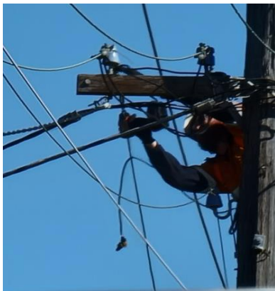
Image showing absence of required Electrical Insulating Gloves or temporary insulation
