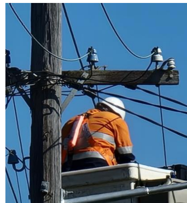
Image showing poor worker body position and no temporary insulation on live LV
