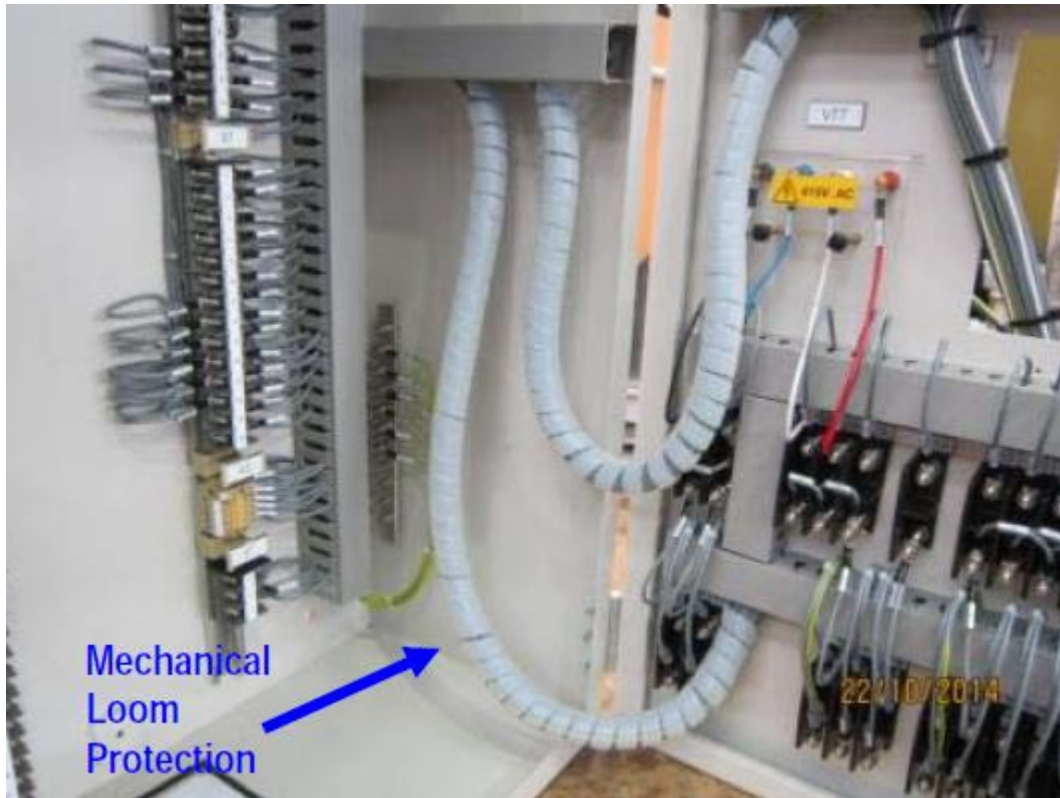
Figure 8 – wiring between panel doors and cabinets
