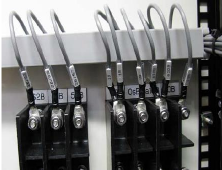
Figure 7 – wiring over ducts
