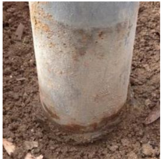
(b) Pole is serviceable
