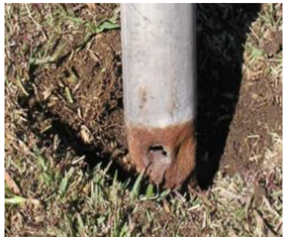
(l) Emergency Line and Defect notice
