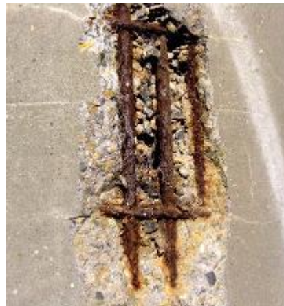
(b) Defect notice
