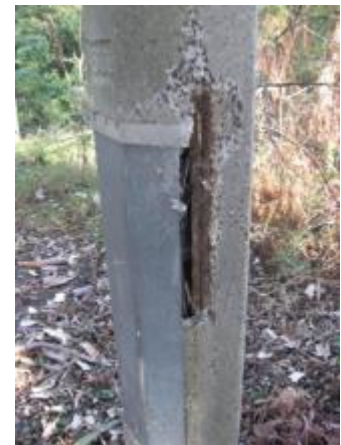
(c) Defect notice
