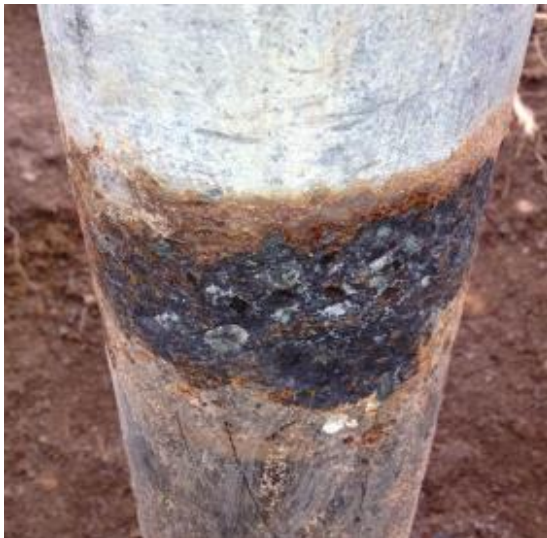
(i) Defect Notice
