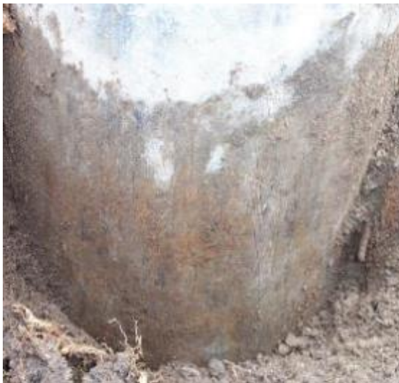
(a) Pole is serviceable
