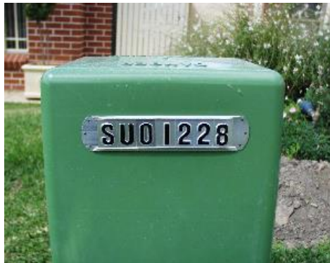
Figure 8.7 - Identification label on a polypropylene plastic pillar
