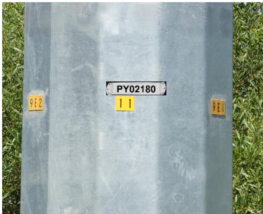
Figure 8.15 – Dual Feeder Pole
