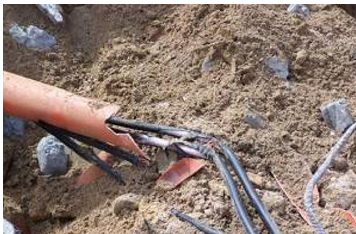
Figure 8: Example of damaged Ausgrid asset
