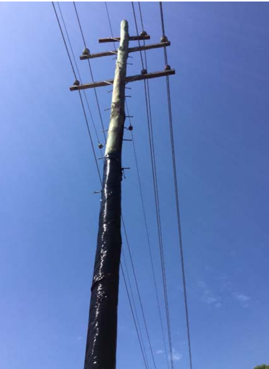
Fire damage and repairs to Ausgrid pole
