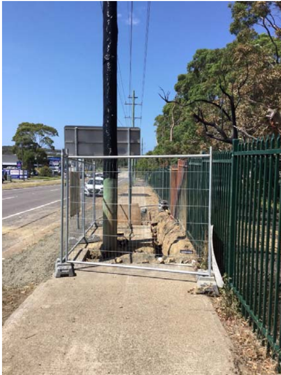
Extent of damage
