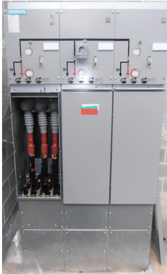
Figure 1 – 8DJH 'RRR' unit.
