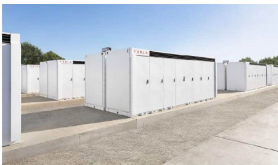
Figure 2-2 Tesla Megapack units (source: Scoping report, AECOM)
