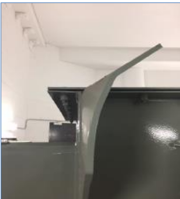
Figure 1: Distorted 10mm thick lifting lug
