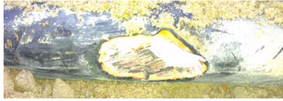
Picture: damaged 33kV underground cable
