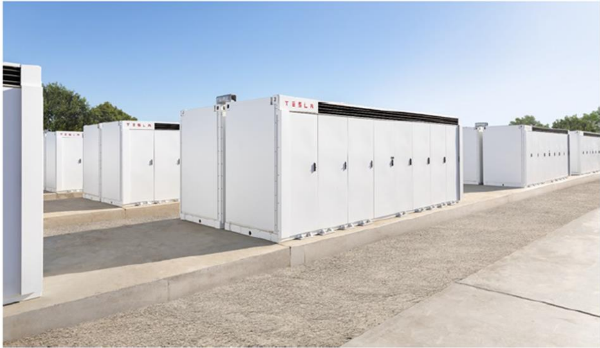
Figure 3-3: A typical BESS site
