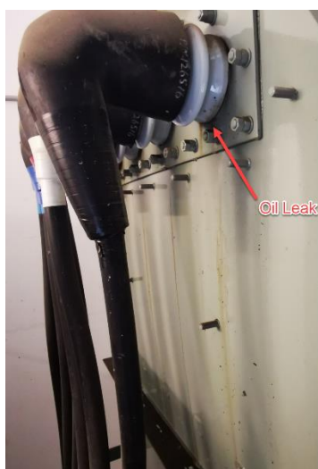
Disturbed LV Bushing Gasket - Schneider 100kVA Tx
