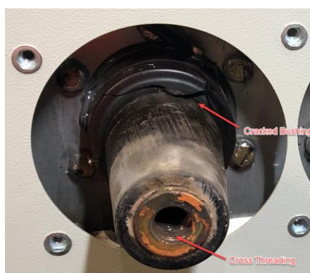
Cracked 11kV Switchgear Bushing - Lucy VRN6a
