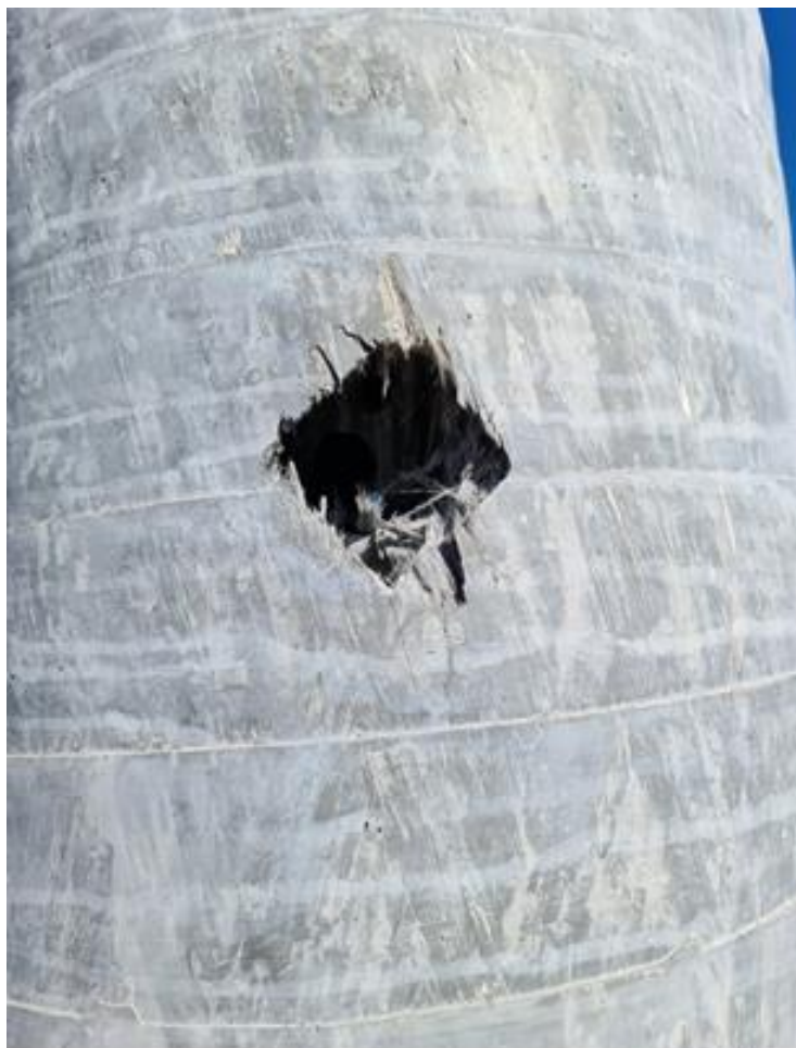
Figure 61 – Damage caused by cross arm king bolt 'pull through'
