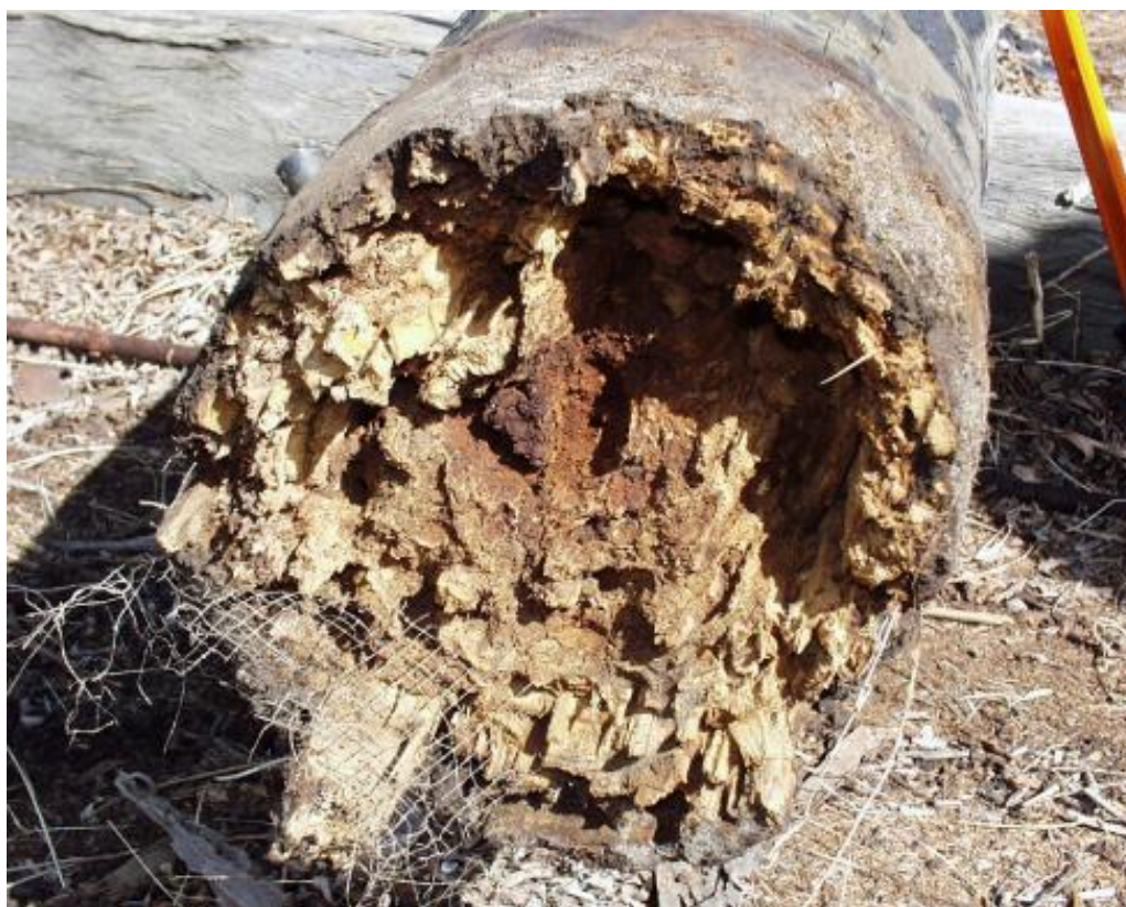
Figure 36 – Glyptotermes Damage Causing Pole Failure
