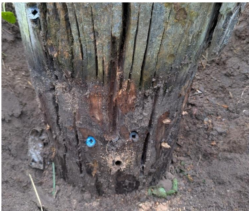
Figure 43 – Ribs on surface which are sound and do not extend significantly into the pole heart
