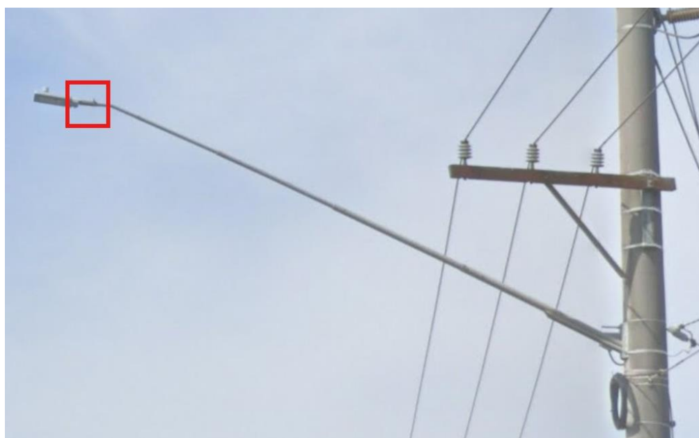
Figure 19 – Example of concrete pole insulating spigot installations
