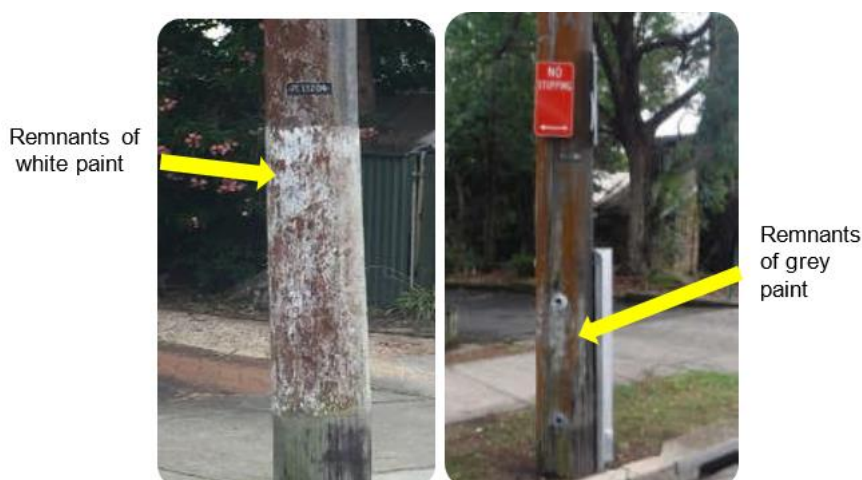
Figure 1 – Examples of Poles with Remnant Friable Asbestos Paint
