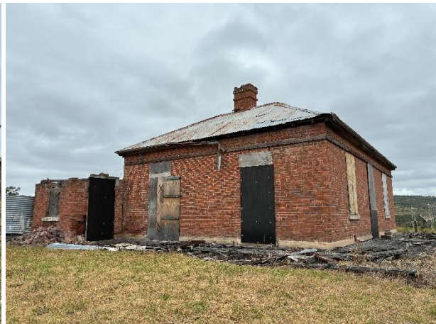
Figure 4-12 West elevation showing damaged timber decking, corroded roof and broken chimney (Source: AECOM 2025)
