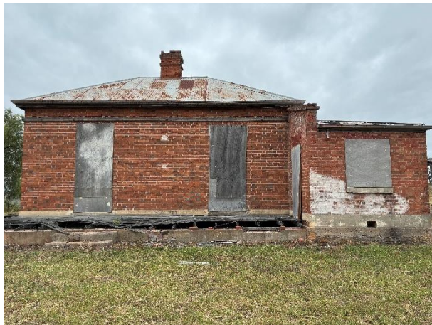
Figure 4-11 East elevation showing damaged timber decking, corroded roof and broken chimney (Source: AECOM 2025)
