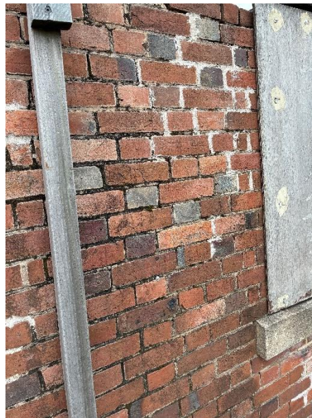
Figure 4-18 Wall with excessive moisture (Source: AECOM 2025)
