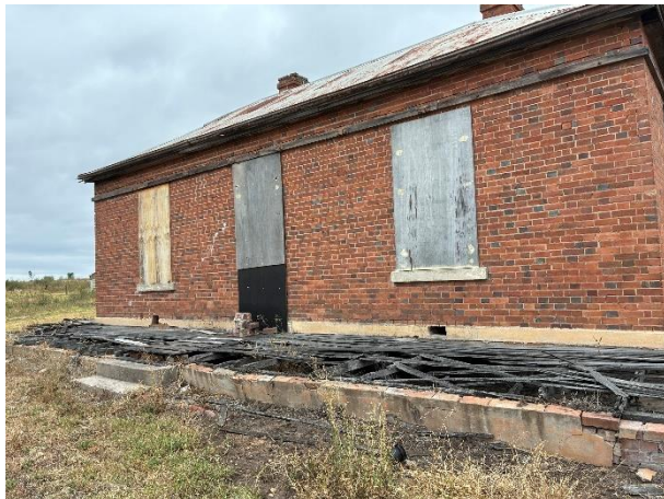
Figure 4-7 North elevation showing collapsed verandah and foundations (Source: AECOM 2025)
