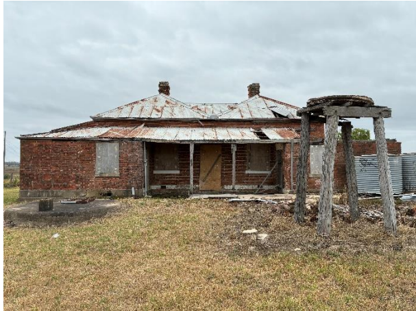
Figure 4-9 South elevation showing further corrosion of roof sheeting, and deterioration of walls (Source: AECOM 2025)
