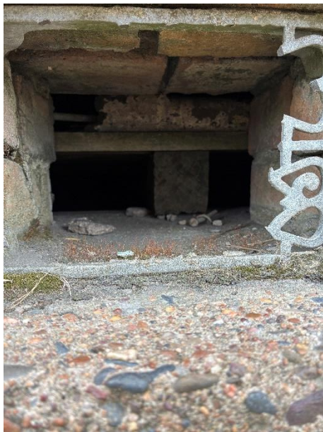
Figure 4-17 Broken steel wall vent showing stone and brick foundations (Source: AECOM 2025)
