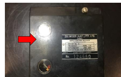
Zellweger – ZEQ relay with asbestos black bituminous casing
