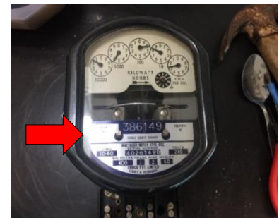
Example of electromechanical BAZ meter with asbestos black mastic
