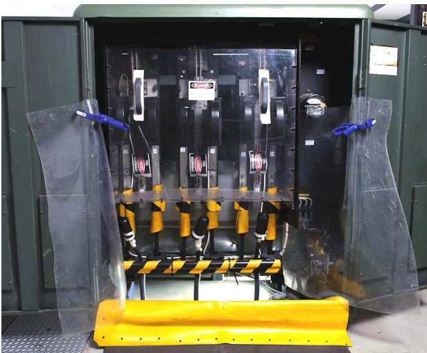
Figure 24 - LV temporary insulating covers and an insulating mat at a kiosk substation
