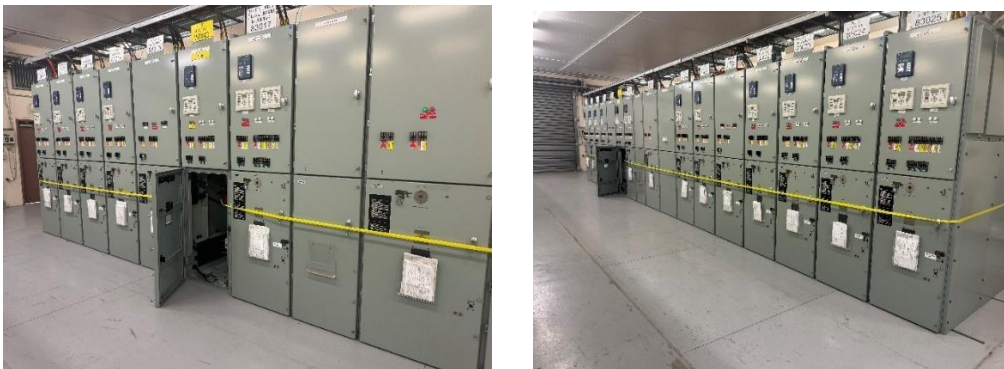
Figure 33 - An example of barrier-out method used on indoor metal-clad switchgear.
