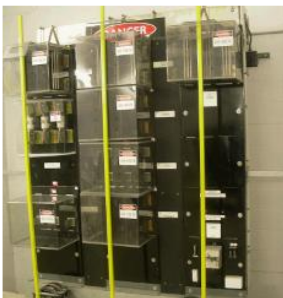
Figure 21 - A screen over exposed LV apparatus in a substation.
