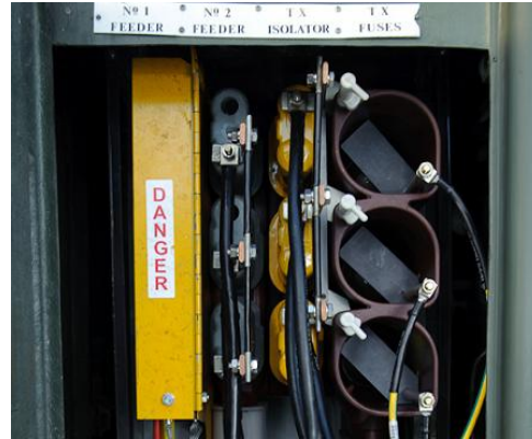
Figure 23 – An earthed screen in place covering live feeder spouts (note the busbar is earthed)
