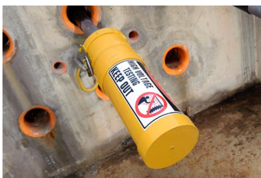
Figure 61 - Lockable cable termination with danger notice
