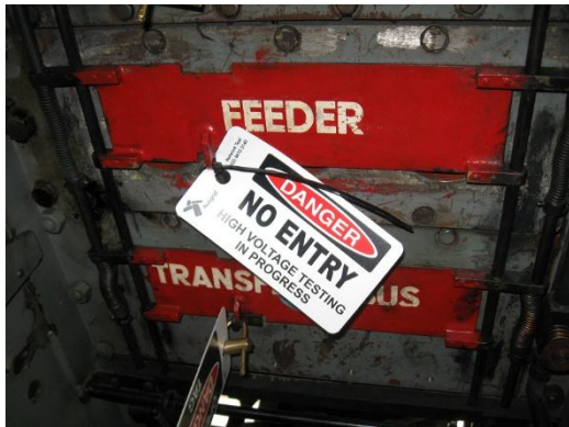
Figure 63 – HV testing tag applied
