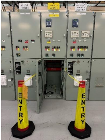
Figure 32 – An example of a barrier-in method used on indoor metal-clad switchgear
