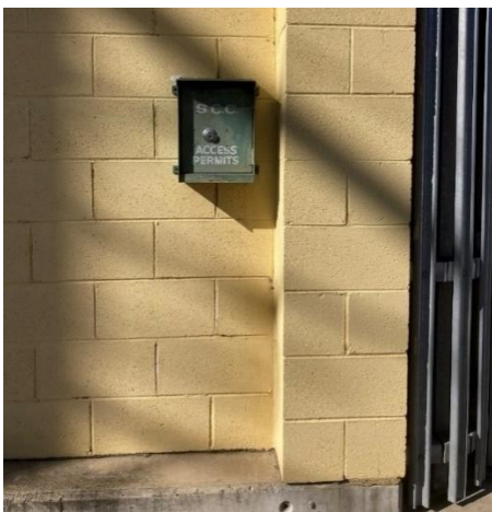
Figure 66 – Permit container on a Transgrid Substation
