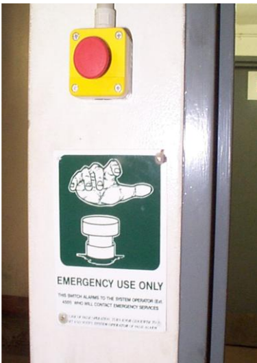
Figure 1 – An emergency switch in a Sydney CBD distribution substation
