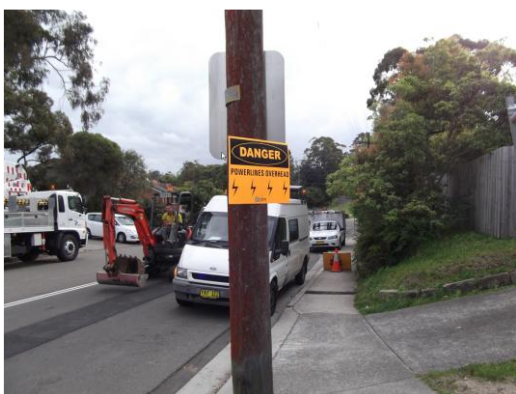
Figure 44 - Temporary 'Powerlines Overhead' warning sign
