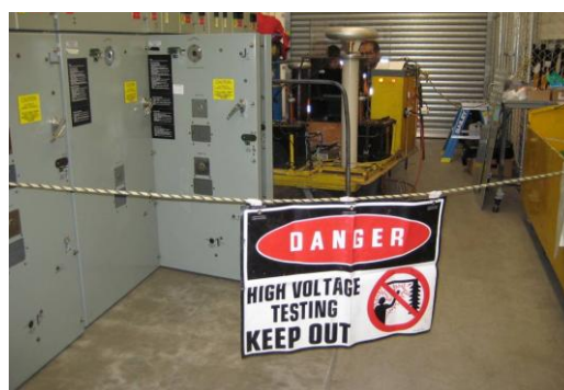
Figure 62 - Black and yellow rope barrier with danger notice
