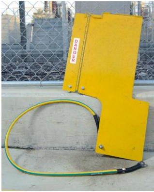
Figure 22 – An earthed screen for Hazemeyer switchgear
