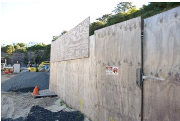
Figure 28 – An example of hoarding used to prevent workers encroaching MSWD
