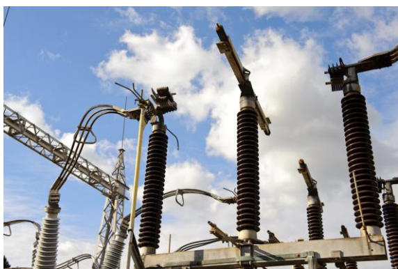
Figure 53 – Open 132kV isolator with closed earthing switch
