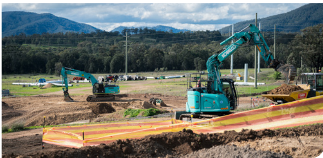
Works at Sandy Creek substation
