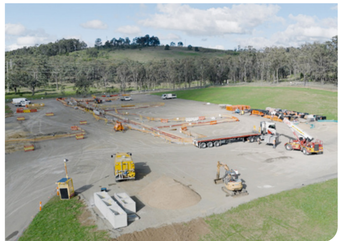
Works at Sandy Creek substation
