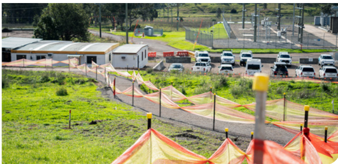
Works at Sandy Creek substation
