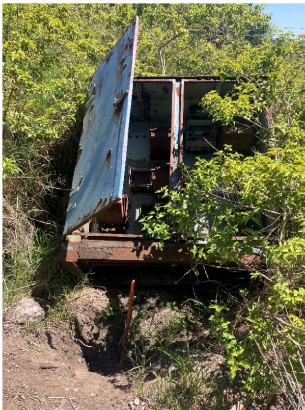
PHOTOGRAPH 9: Old electrical box located in the northwestern corner of the site.
