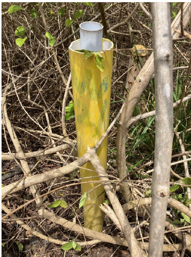
Groundwater well, BHW2/1, situated in the northeastern corner of the site.
