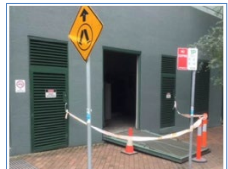
Figure 2: Panel fell onto footpath
