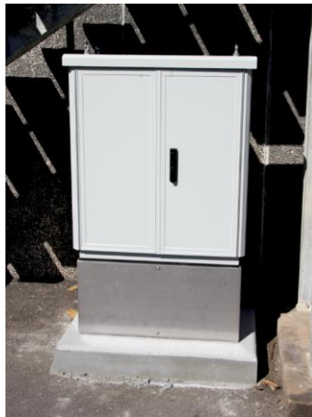
Figure 12 – FDA – Fibre distribution ancillary panel
