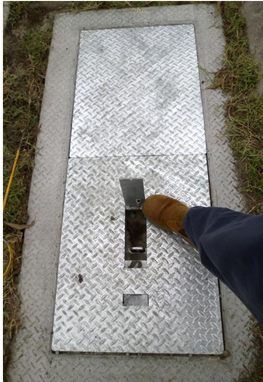
Figure 9 – Telecommunications pit (padlock removed)
