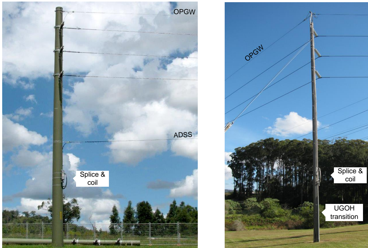
Figure 10 – Examples of Ausgrid aerial cable, splice and UGOH installations
