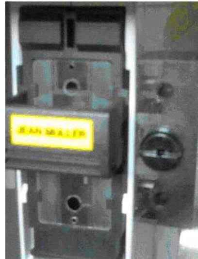
Figure 47 - Moulded plastic component in the side of the switchgear module
