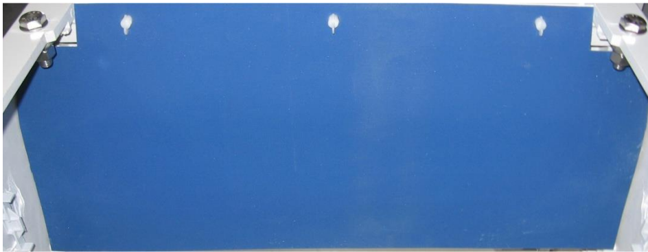
Figure 19 - Insulating mat covering the neutral bar
