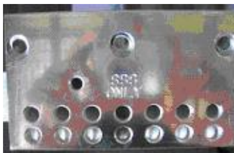
Figure 40 - Active terminal block (removed from cabinet, no grub screws installed) depicting “SSS ONLY” marking.
