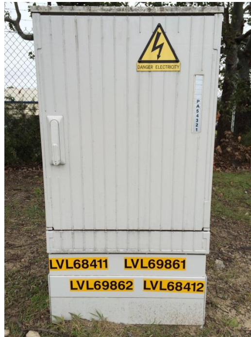
Figure 103 - Example of “link number” labels affixed to the top front cover of the base unit in the same order as the links are positioned inside the cabinet
