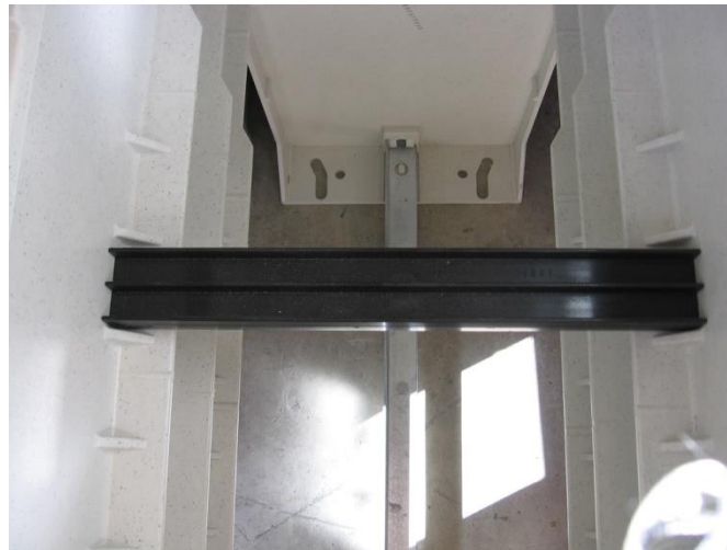
Figure 27 - Base Unit support bar installed in position. (Viewed looking down into the direct buried base unit.)
