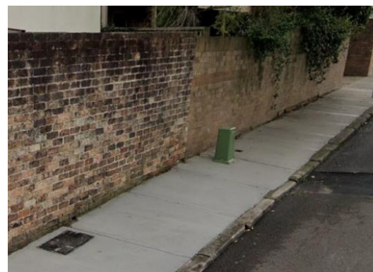
Fig B6 - Unacceptable – Narrow footpath, marginal on adequate width and contrast. A commercial pillar would be suitable for this location.
