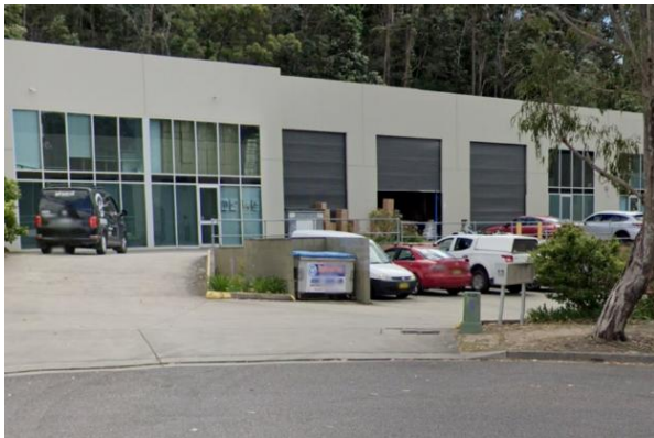
Fig B30 - Unacceptable – Low pillar with inadequate setback from commercial driveway and significant risk of vehicle impacts.
