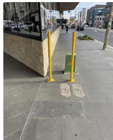
Fig B24 - Unacceptable – Low distribution pillar too close to building corner. A commercial pillar would be suitable using clearances per Table 1.
