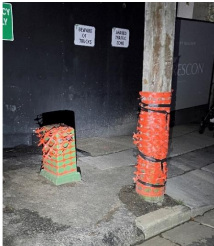
Fig B7 - Unacceptable – Low pillar is opposite existing pole and further impedes narrow footpath.
