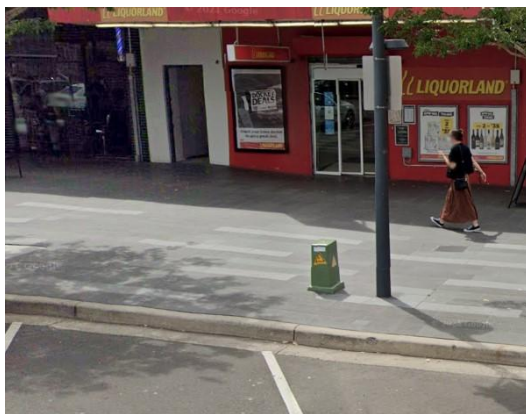
Fig B15 - Acceptable – Low pillar, but in line with other fixed assets and within 1m.
