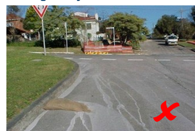
Saw-cutting slurry has not been contained effectively
