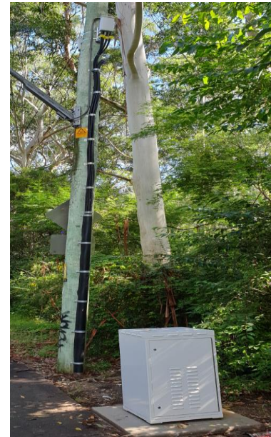
Small Cell Antenna with ground mounted equipment cabinet
