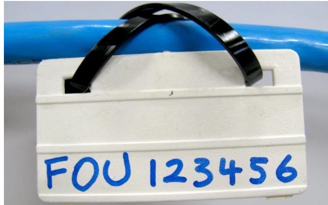
Figure 2 – Telecommunications cable label example
